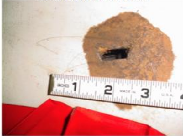
BEAVER VALLEY UNIT 1 LINER HOLE
