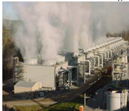
Figure 5. 40-cell Plant Yates cooling tower 25
