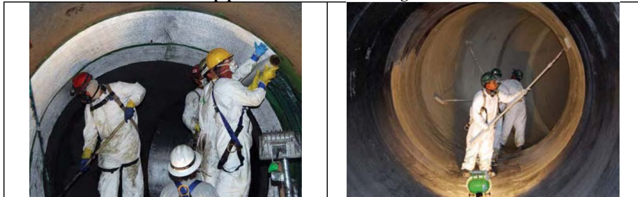
Figure 3. Application of CFRP to interior walls of existing 10-foot diameter circulating water pipe at San Juan Generating Station 27
